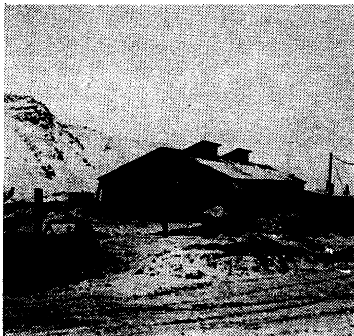
Plate 1.6 The pump stations were generally 30 to 35 miles apart. Pump Station No. 6 was at Mile 208E and is depicted here while under construction (photo by R.S. Finnie).
