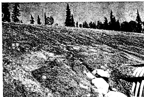
•large fills offer the potential for shoulder erosion
